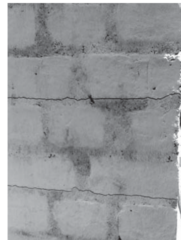
Fig. 6 Observed failure pattern of the half-brick thick masonry wall
